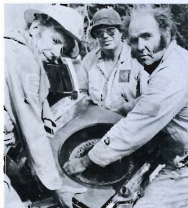
Pictured above from left: John Savage, John Luscombe and Ken Ross, fit the repaired radiator to their fire truck.
