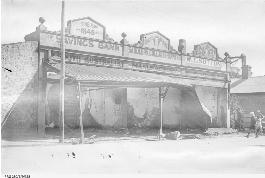
State Library of South Australia - Fire damage at Simon's Depot, Balaklava, Damage caused by fire at Simon's Depot, Balaklava to the premises of a Savings Bank of South Australia, Simon's saddlery, and W.G. Sutton's greengrocer. Approximately 1918. Part of Searcy Collection.
